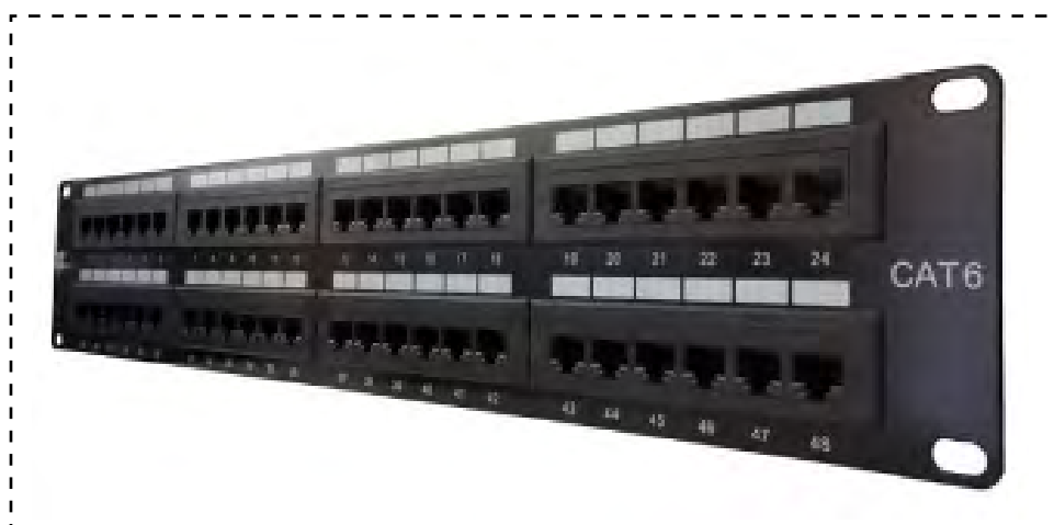
Figura 1.2. Patch Panel de 48 puertos
